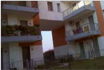
Visual image of the heat leaking from the building.
