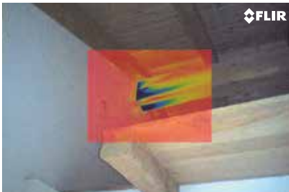
Air leak during blower door inspection, Picture in picture image.
