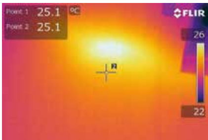
This hot water leak clearly shows up in the thermal image.
