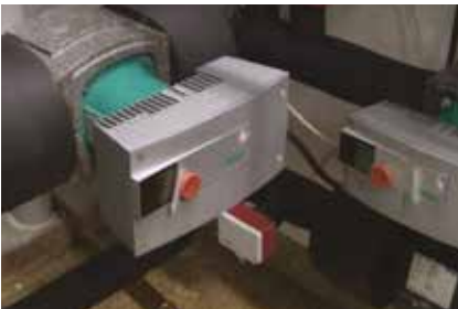
Thermal image and visual image of an electric water pump.
